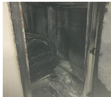
Original fire-damaged AHU
